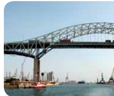
The aging Gerald Desmond Bridge in Long Beach wears a "diaper" to catch falling debris.
